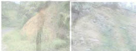
Fig. 6. a) Soil slide, b) Debris fall
