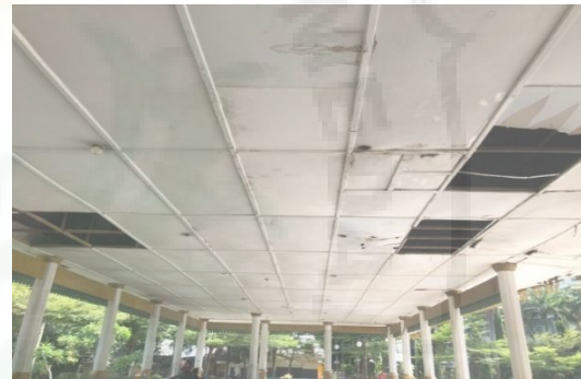
Fig: Damage to the roof of the Tribune and Pandopo Merdeka Square, Source: Doc. Private, 26 June 2021
