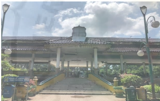
Fig: Damage to the Canopy and Floor of the Tribune/Pandopo Merdeka Square Staircase, Source: Doc. Private, 26 June 2021
