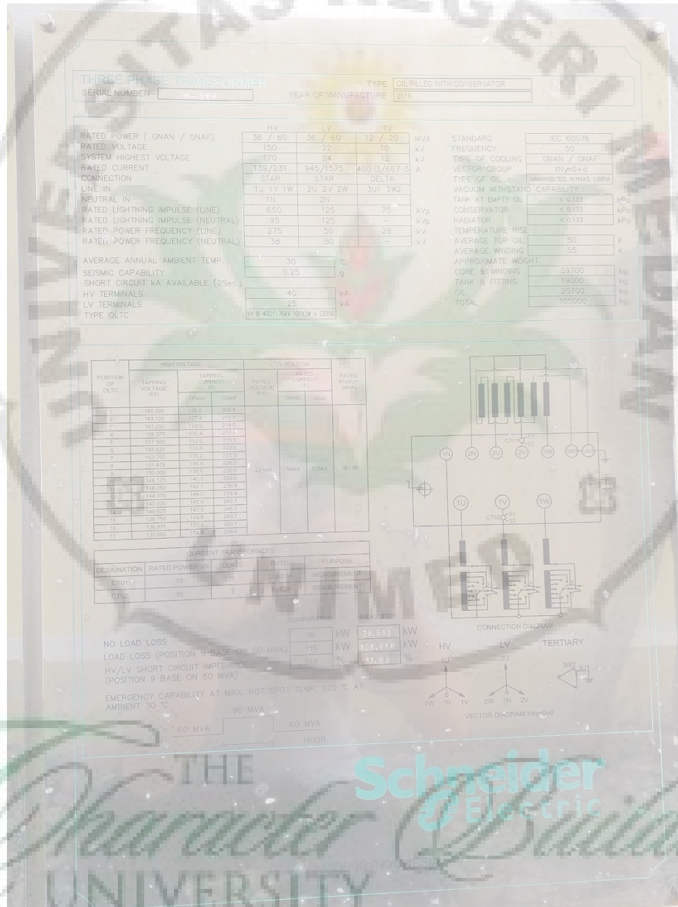
Gambar 7. Nameplate Transformator Daya 3 Schneider GI Sei Rotan
